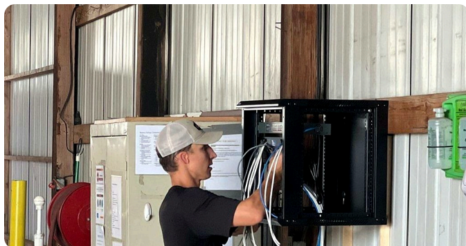
Clean, labeled network racks make systems reliable and easy to service.
