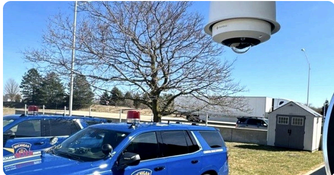
PTZ camera installation for the Michigan State Police.
