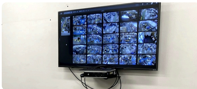
A 12-camera live view on a Michigan warehouse system we installed.
