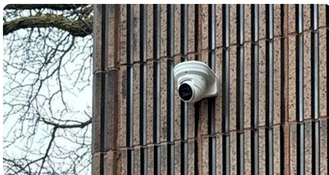
An exterior dome camera covering a building entrance.
