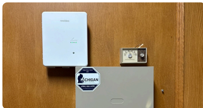
A monitored alarm upgrade we installed at a Royal Oak church.
