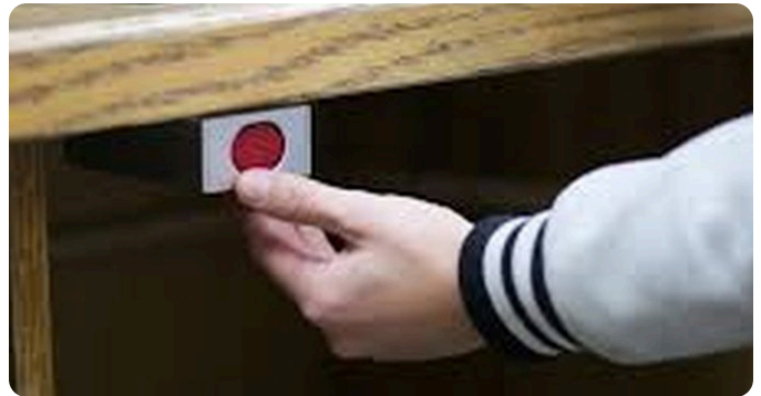
A discreet panic button installed under a front desk.
