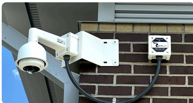
A PTZ camera and “Protected by” sign: deterrence you can see.
